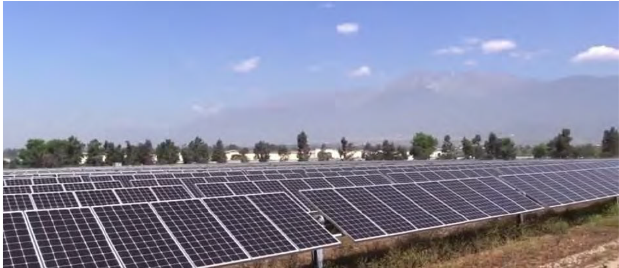
Solar panels at the Caltrans Traffic Management Center in Fontana, District 8
