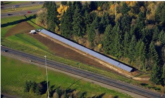
Oregon DOT-installed solar array at the interchange of I-5 and I-205 near Portland
