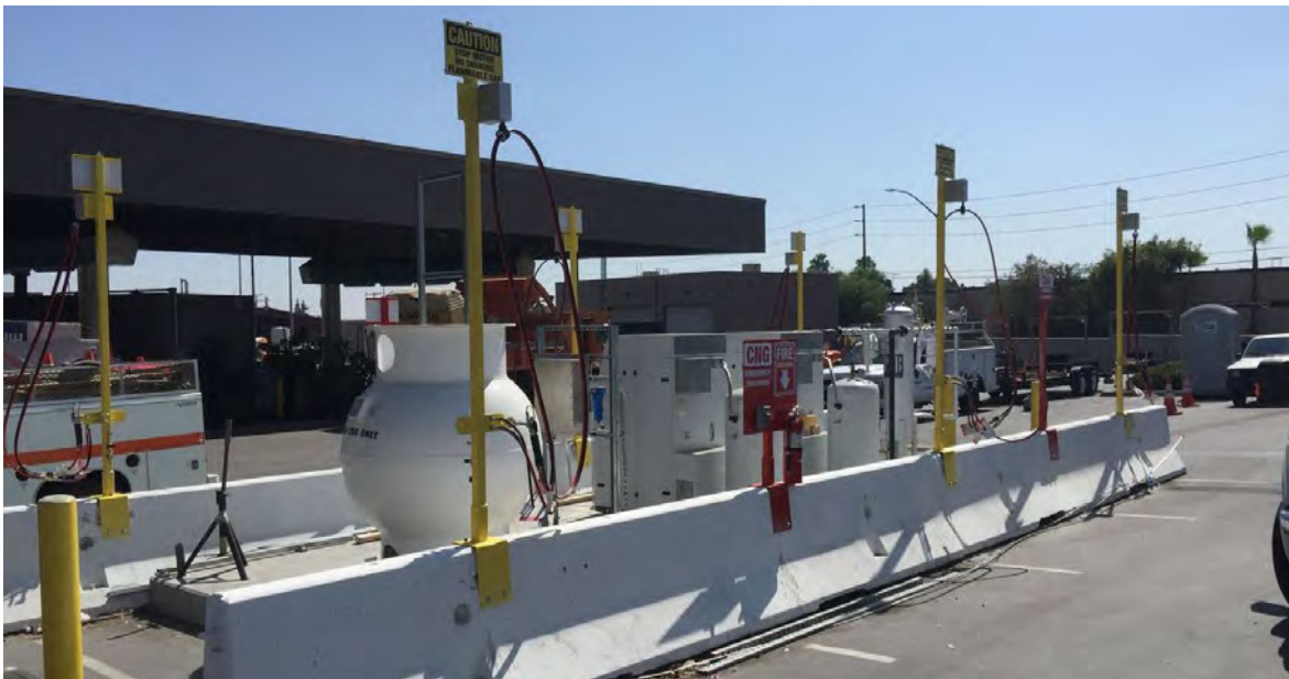
CNG Fueling Infrastructure at Caltrans Foothill Maintenance Station, District 7
