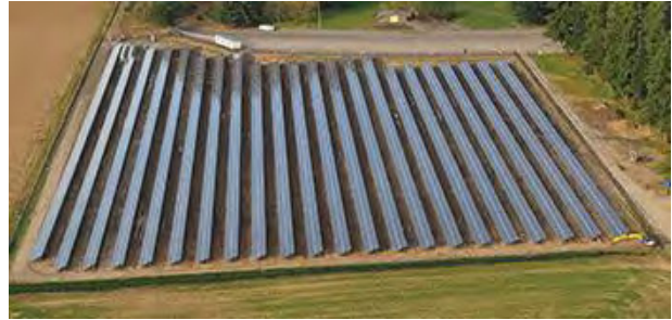
Oregon DOT-installed 1.75 MW solar array at the French Prairie Rest Area on I-5
